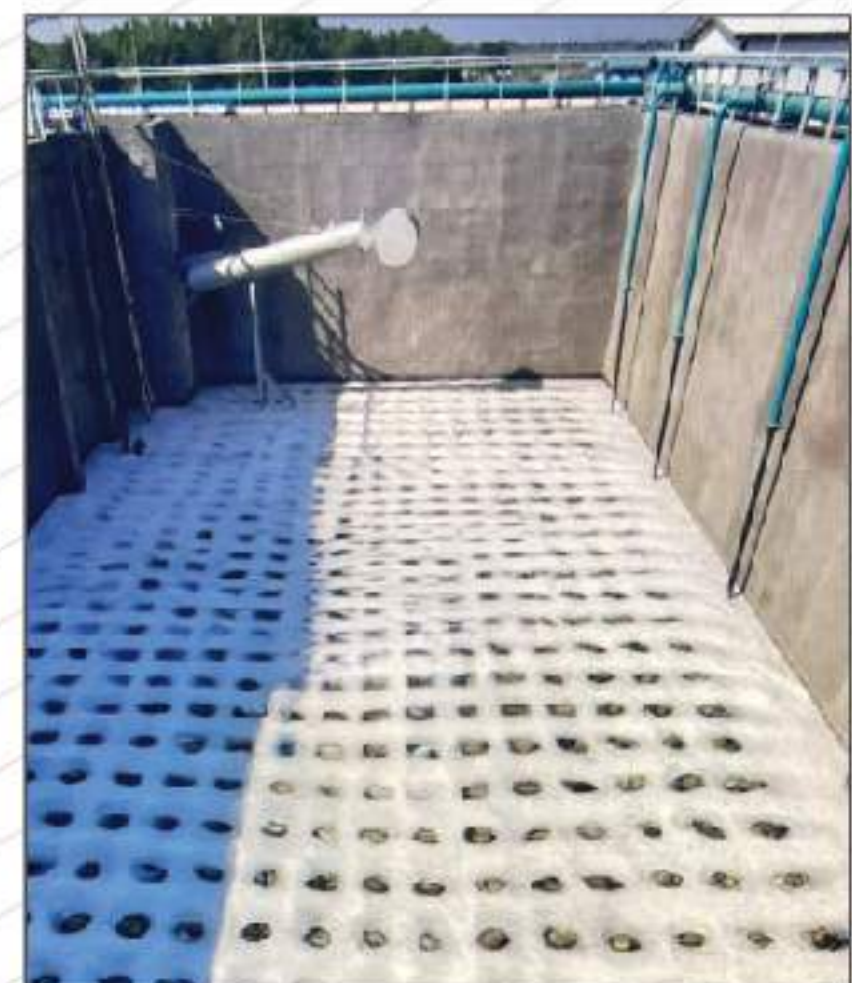
WASTEWATER TREATMENT PLANT TEXTILE INDUSTRY
