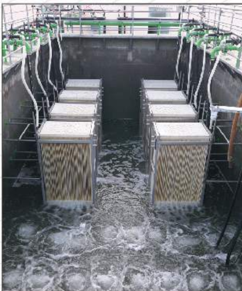
WASTEWATER TREATMENT PLANT GREY WATER
